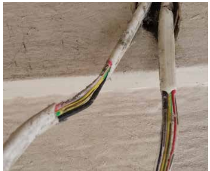
Here is an example of the damage rodents can do to electrical wiring, exposing conductors, which can lead to fire or electric shock
