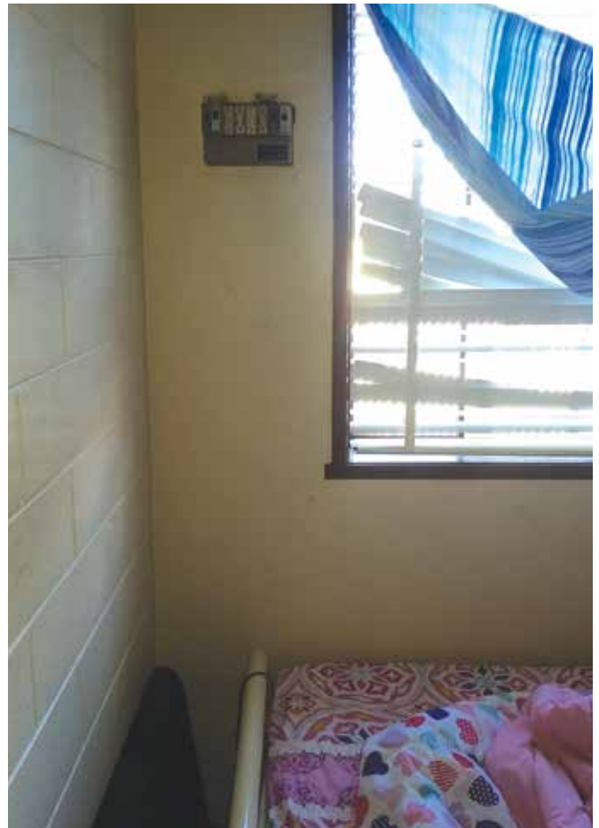
Here's a great example of what not to do in a rental property – a switchboard located in a child's room reachable from the bed. No tools were required to remove the fuses that then exposed live copper terminals
