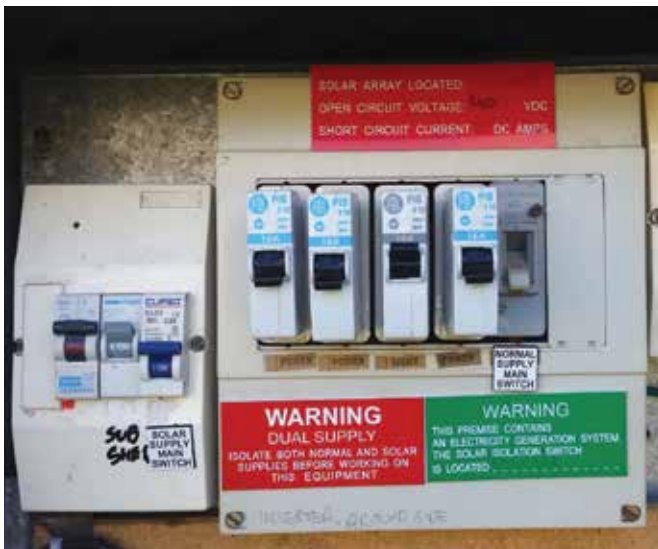
An 'old-school' style switchboard with DIY circuit breakers. This particular switchboard had a solar installation installed and yet preventative safety measures were not taken to upgrade it to today's safety standards
