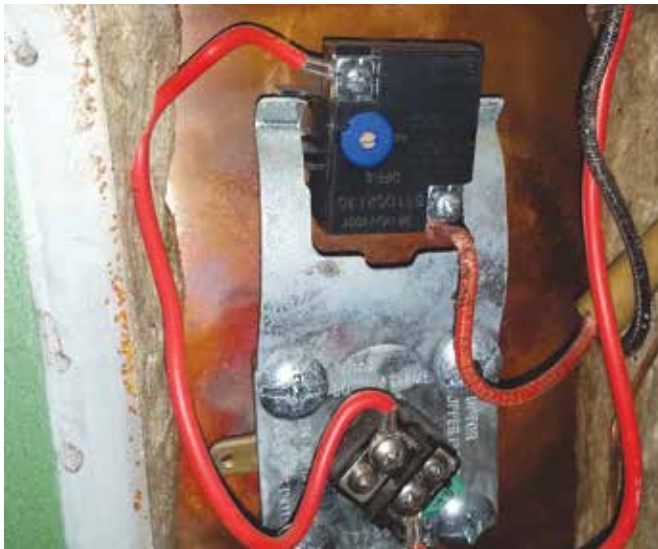
This hazard was identified during an electrical audit – an electric hot water service with its protective cover removed. The service was located in a cupboard where children's sports goods were stored, exposing them to the risk of electric shock
