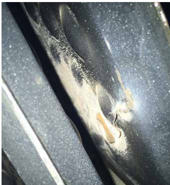
A crack in a heater revealed alarmingly high carbon monoxide levels escaping into the living space of this home
